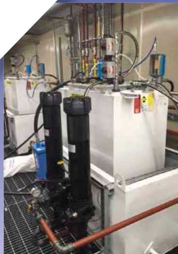
Hydraulic reservoirs with LMD 431 in-line duplex filters
